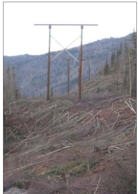
Top, CVEA right-of-way before clearing maintenance Above, CVEA right-of-way after clearing maintenance
