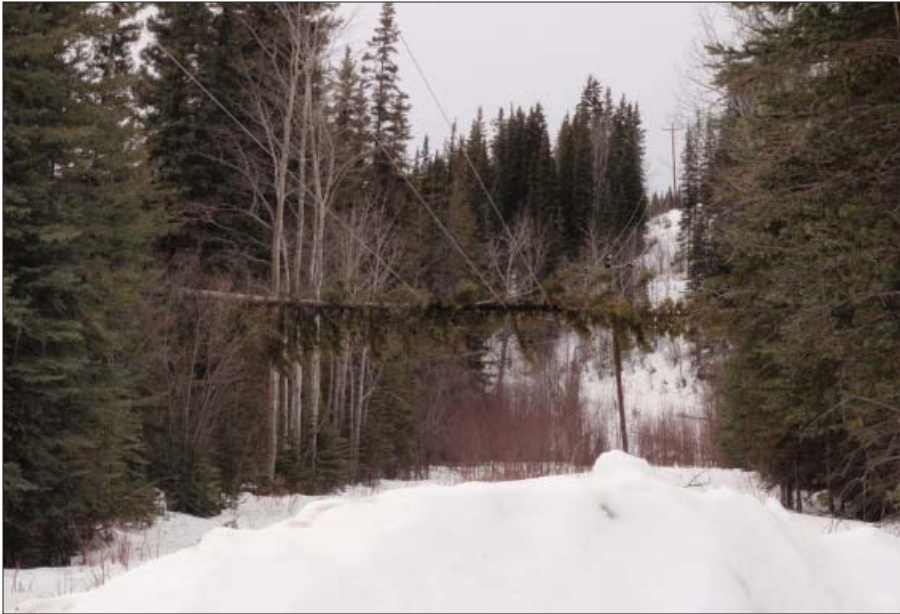
Above, a tall tree from far outside CVEA's right-of-way in the Copper Basin, fell into the power line
